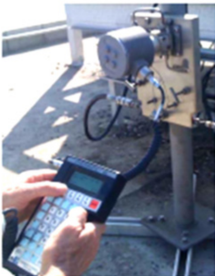
Figure 5: RDC-CI Chemical Data Logger—Retrieving Data with an RCS CheckMate
