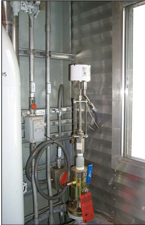
Microcor Transmitter and Retractable Probe in Field Installation
