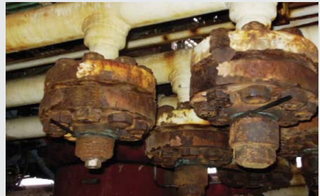
Unmaintained Well Bay - No Double Isolation
