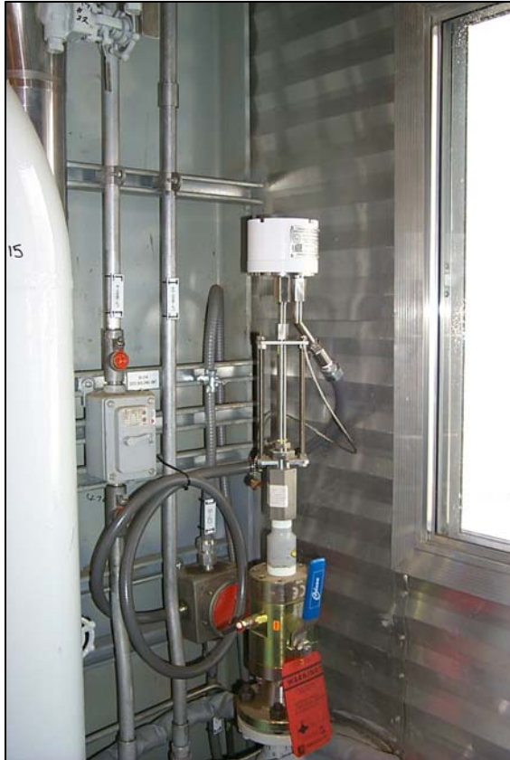
Microcor Transmitter and Retractable Probe in Field Installation
