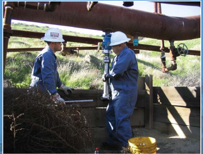
Retrieval of COSASCO® Coupons Under Pressure
