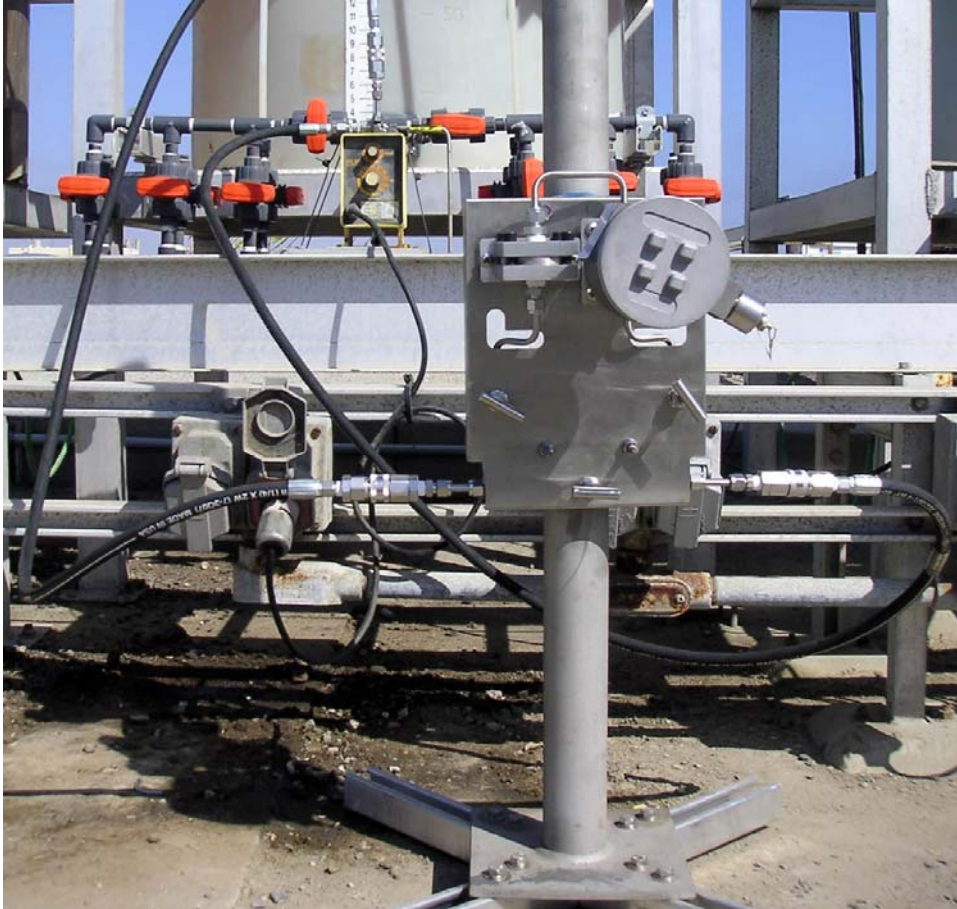
RDC-CI shown in the field installed with flexible connection hoses
